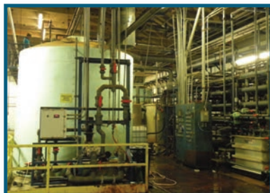
Using the right amount of fresh water vs. recycled water is critical to controlling consumption.
